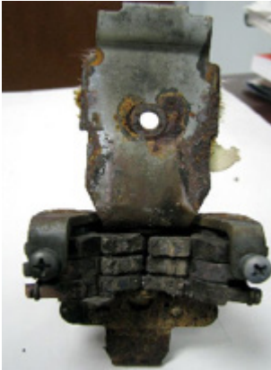
Fig 28: Circuit breaker corrosion
