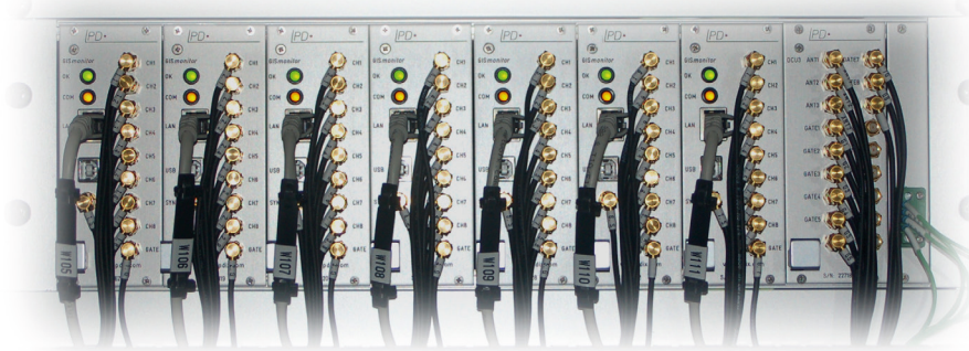
Figure 12: GISmonitor built into a 19-inch rack
