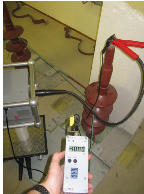
Figure 58: CAL1B connected to MV cable (on-site)
