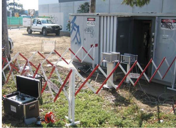
Figure 4: MV cable testing on-site
