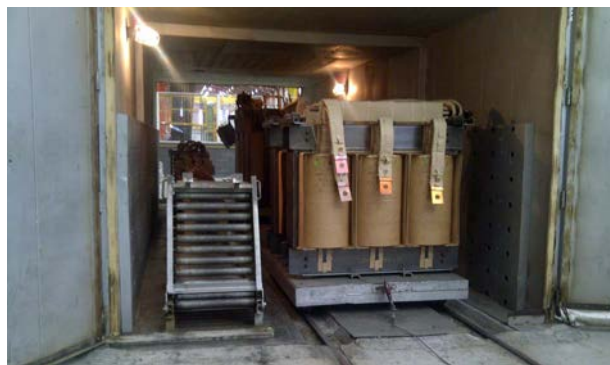
Fig. 1 Location of the experimental 5 MVA transformer's active part inside the oven
