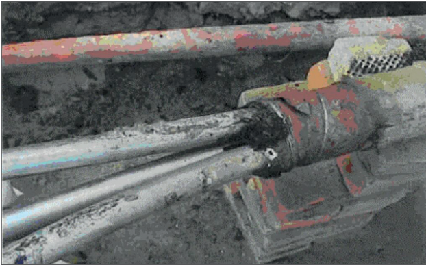
Corrosion on the outer sheath and the building of holes in the lead sheath
