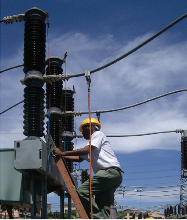
Circuit breaker grounded during preparation for timing test
