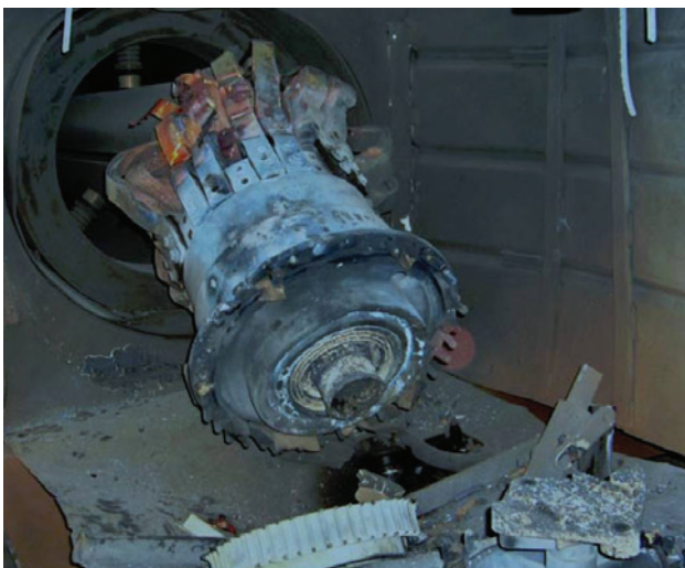
Generator circuit breaker failure
