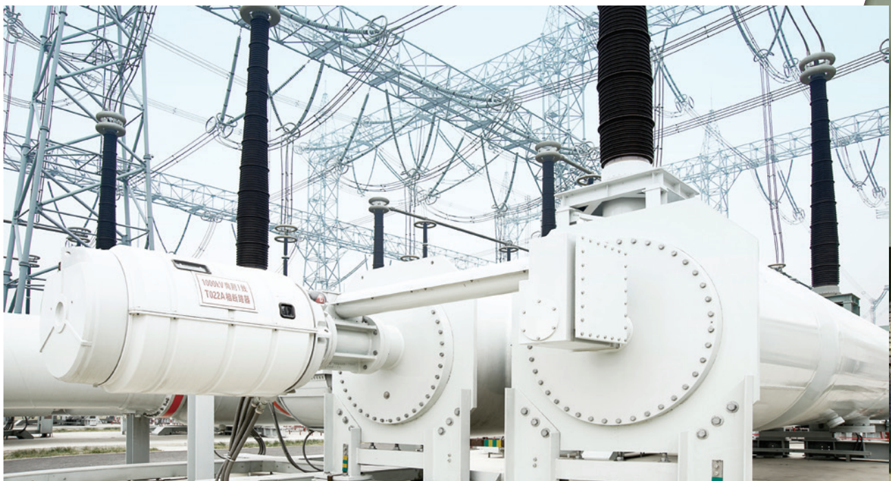
Circuit breaker, 1000 kV
