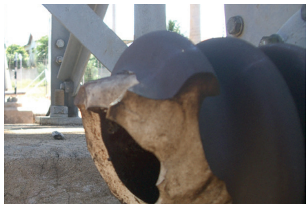
A distribution circuit breaker pole totally damaged by explosion.
