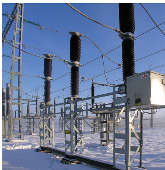
Live tank circuit breaker
