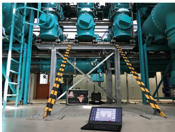
Figure 3.3: GISmonitor Portable installed on a GIS
